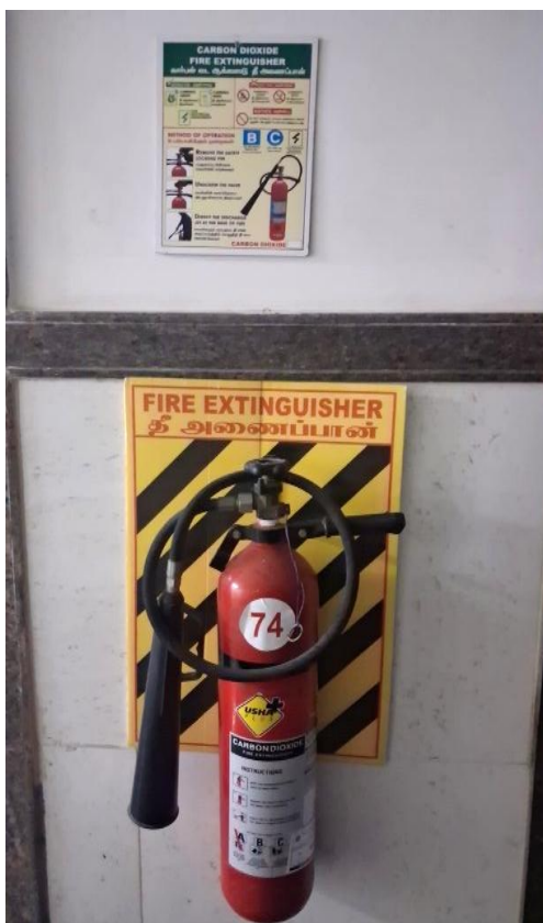
CO 2 – FIRE EXTINGUISHER
