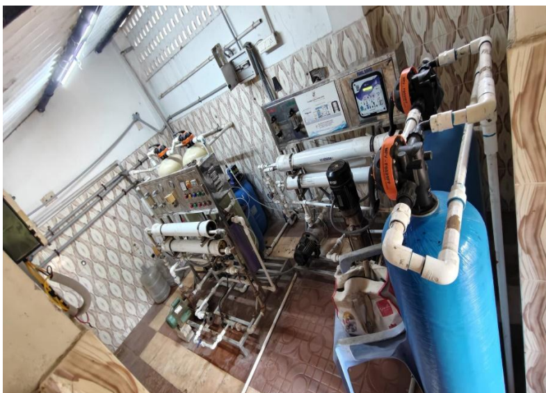
Reverse Osmosis Plant
