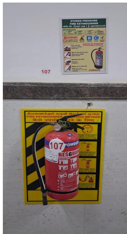
DRY CHEMICAL FIRE EXTINGUISHER
